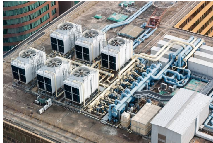
HVAC System Audit
