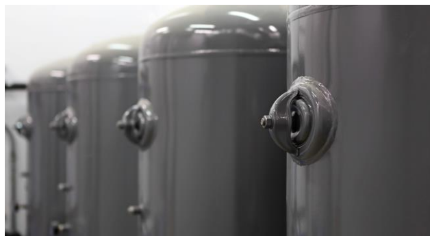
Compressed Air System Audit
